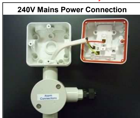
240V Mains Power Connection
